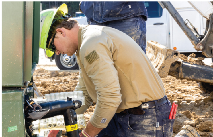
ELW graduate, Austin Hewette, tackles an underground job in Goose Creek during his apprenticeship.
